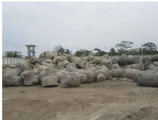
Construction Material without Caution Tape
