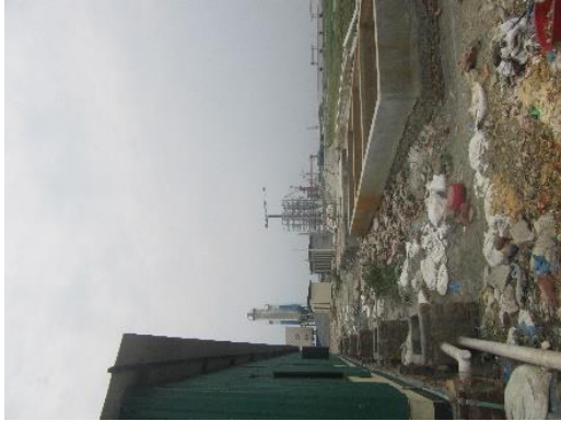
NDE Employees' labor Shed Waste Condition
