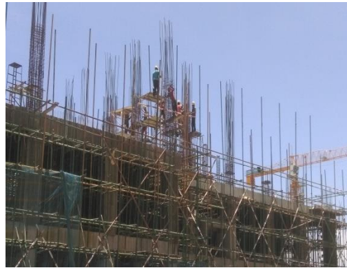
NDE Workers without PPE during working at height
