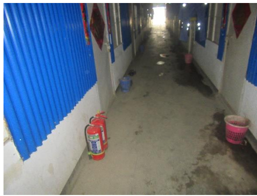
Fire Extinguisher in NEPC Subcontractor Labor Shed
