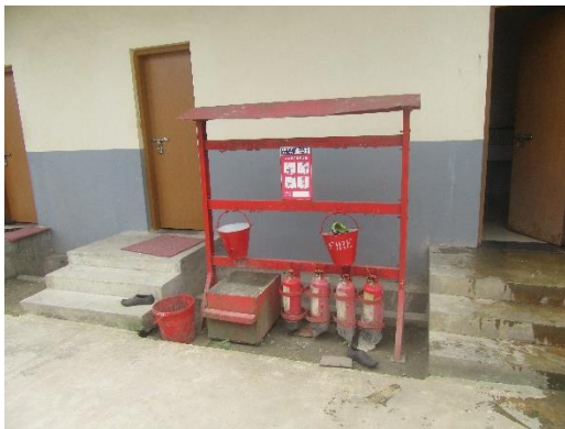
Fire Extinguisher in Project Site
